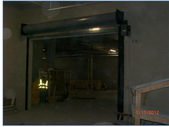
Coiling doors at secured parking
