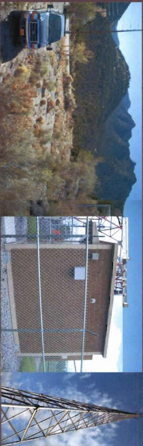
Communication Shelter, 30 Ft. Tower and Communication Equipment
