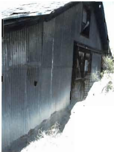
Sediment impacting a historic building at the Coal Mine Museum
