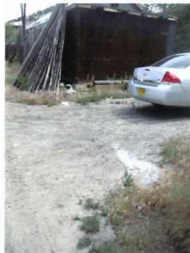
Poorly maintained culvert at Ice House Road
