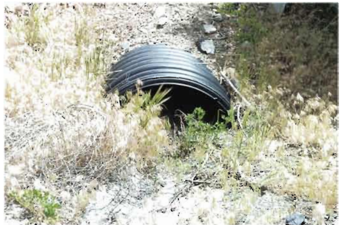
Culvert in arroyo impaired by sediment
