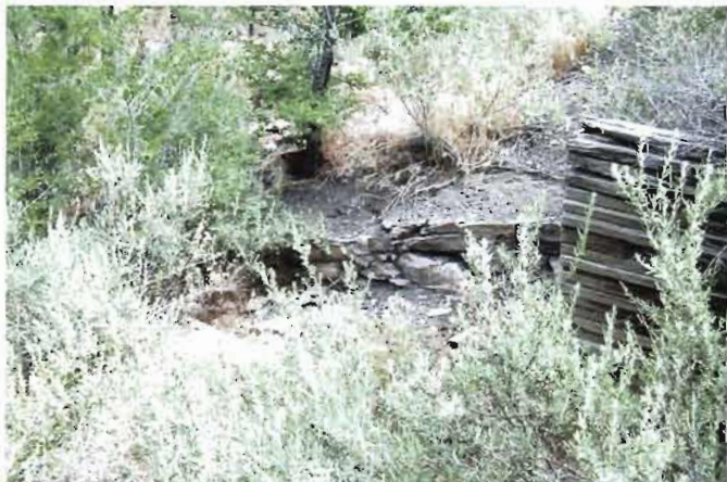
Damaged and abandoned wood flume below Ice House Road
