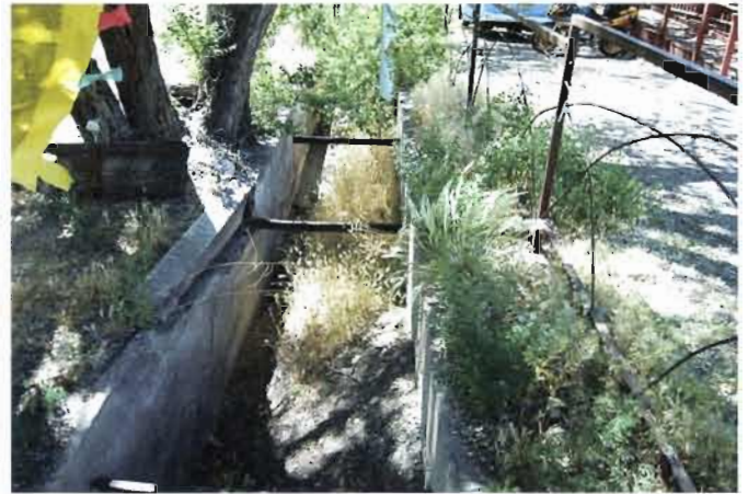
Existing concrete flume. Note sedimentation and conditions.
