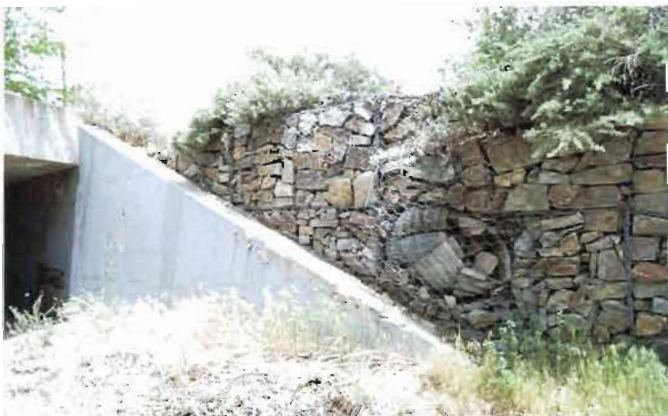
Abandoned culvert in gabion structure at NM 14 crossing
