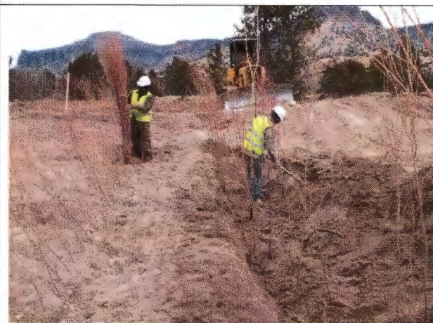
A 0.3-acre willow wetland was constructed in an area formerly dominated by non-native saltcedar and Russian olive trees.
