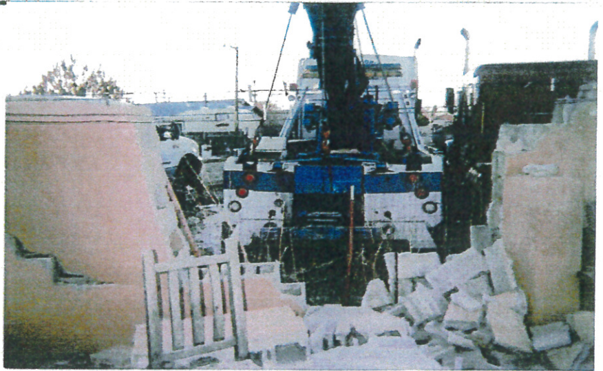
Pictures 1-3: Damage to our privacy wall after Anaya tapped and backed into it creating a 23 foot gap, plus other property damage.
