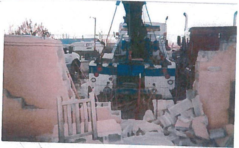
Pictures 1-3: Damage to our privacy wall after Anaya tapped and backed into it creating a 23 foot gap, plus other property damage.
