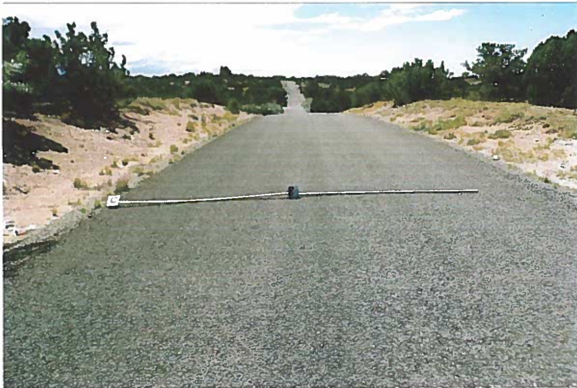
Camino Peralta at top of rise between Terra Bella gate and Camino Espejo, looking south. Road is 17 feet wide.
