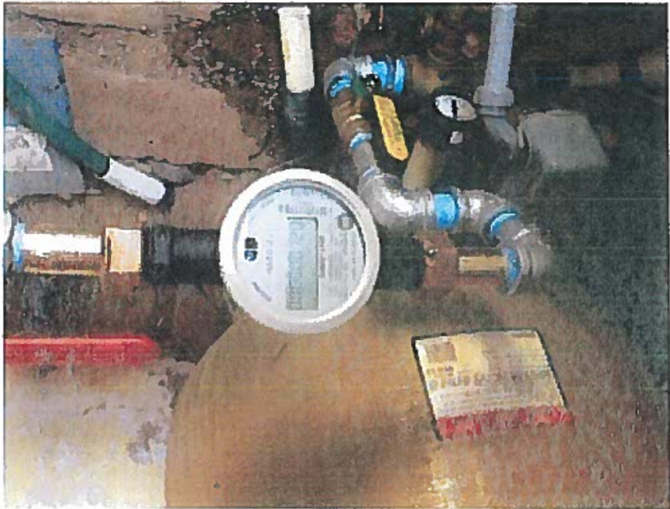
Initial Meter Reading on Date of Installation (Meter Previously Used) 5/1/2014 120 gallons
