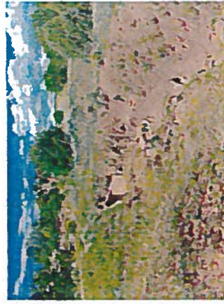
Poorly designed culverts and road drainage systems contribute to erosion and ecological degradation throughout the Basin.
