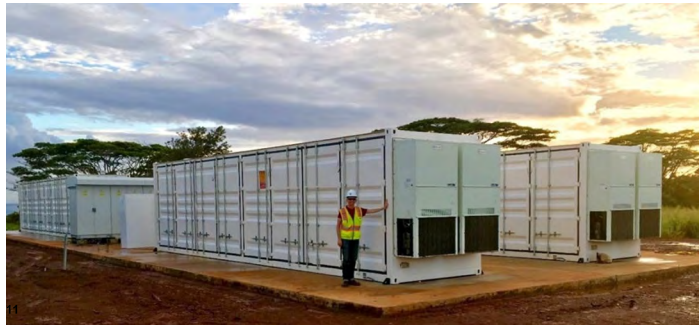
Representative image from earlier containerized BESS solution
