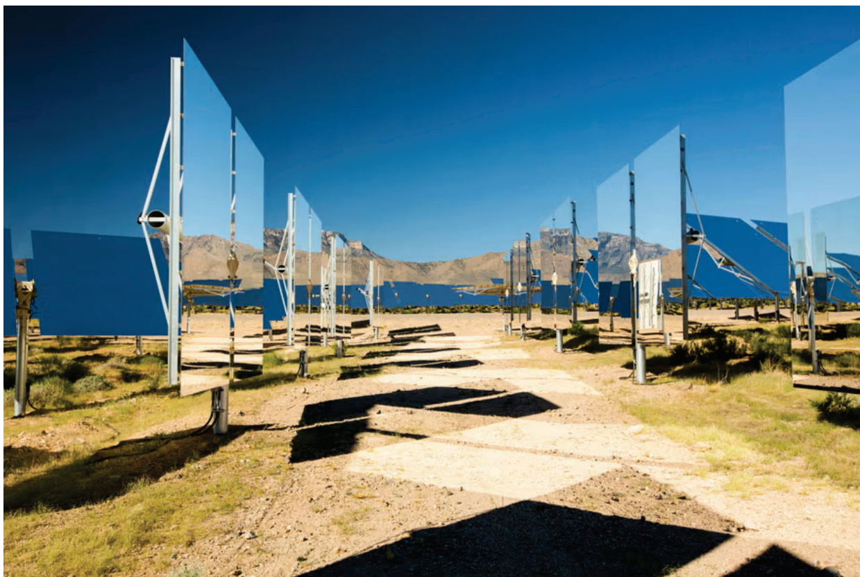
Heliostats at the Ivanpah solar thermal power plant in the Mojave desert. Photograph: Ashley Cooper/Alamy
