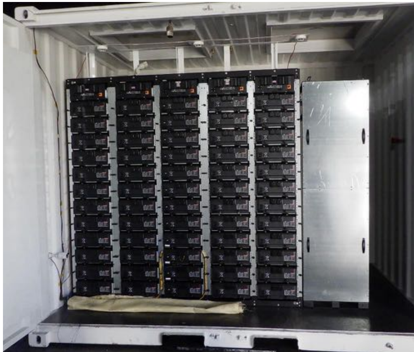
Figure B2 – Photo of Unit and BCP Box
