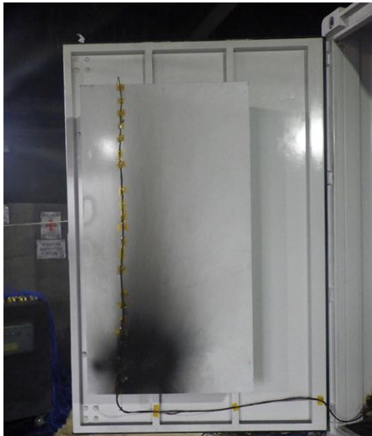
Figure E2 – Photo of the door with Chiller box enclosure and thermocouple arrays after the test
