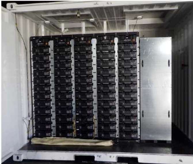
Figure 1 – Picture of the units in the container
