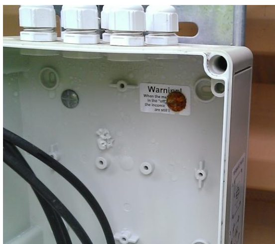
Figure 9: Rear of isolator enclosure drilled through for mounting screws. Note that the screw on the right hand side is rusty, indicating water ingress.
