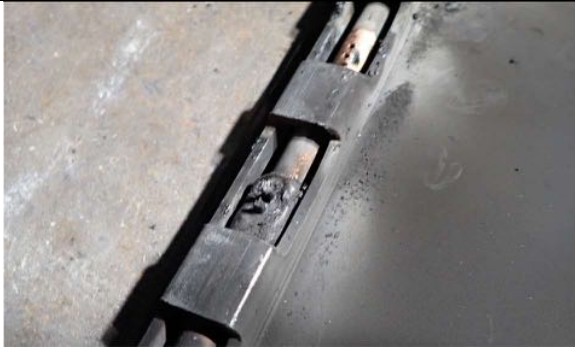
Post Test – View of the NOVEC Piping
