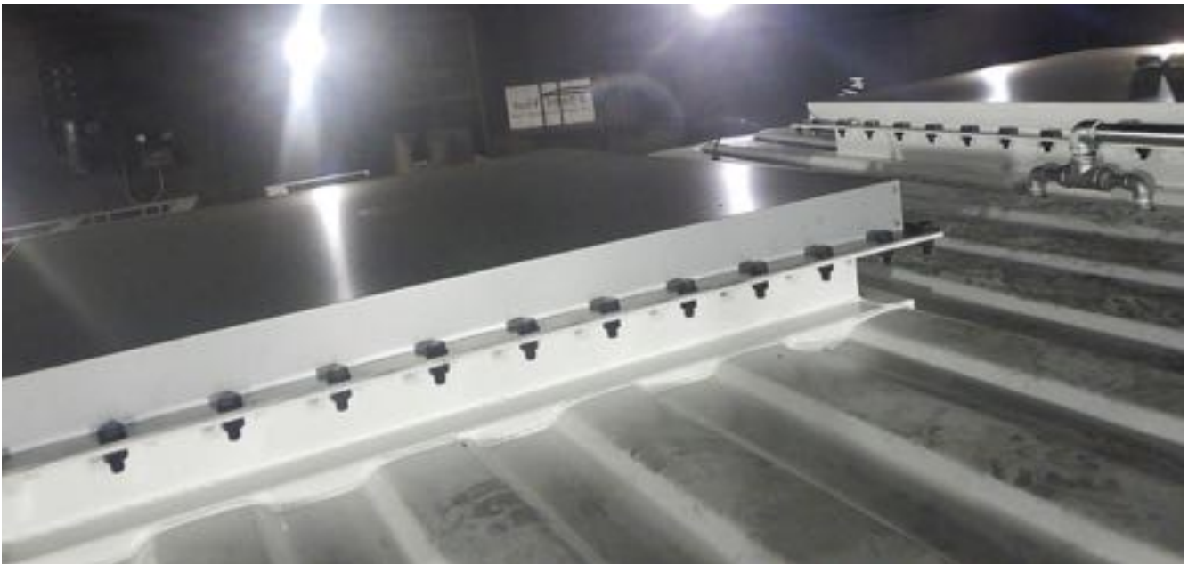
Figure F7 – Photo of the deflagration panel on the ceiling (taken from outside of the container)
