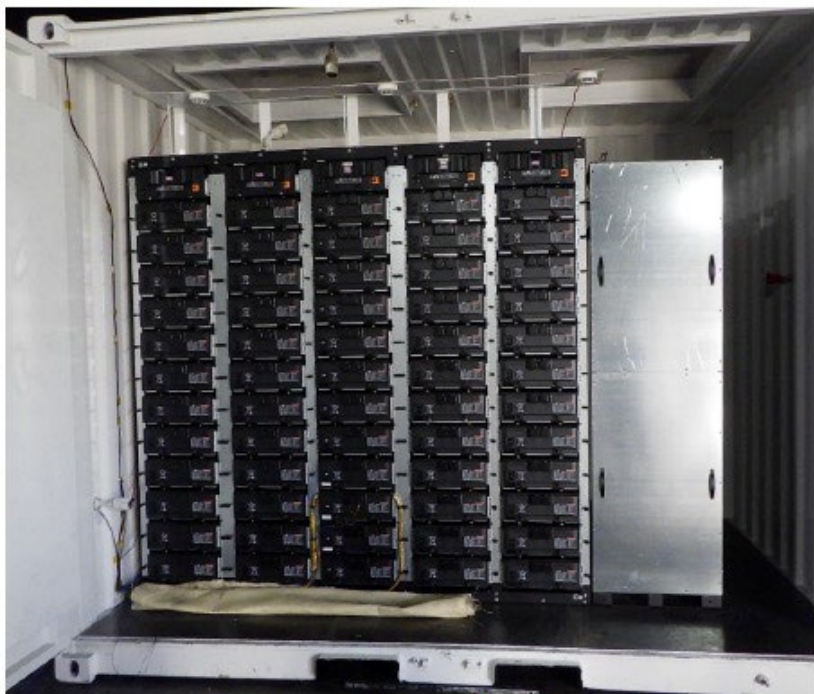
Figure 1 – Picture of the units in the container
