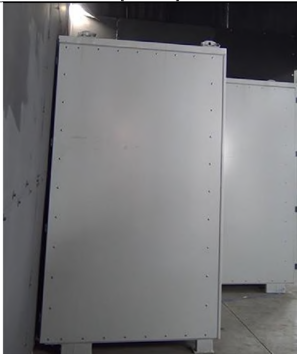
(c) Initiating cell thermal runaway [00:41:42]
