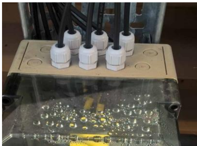
Figure 8: Water can be seen inside this enclosure, even though only one cable passes through each gland.
