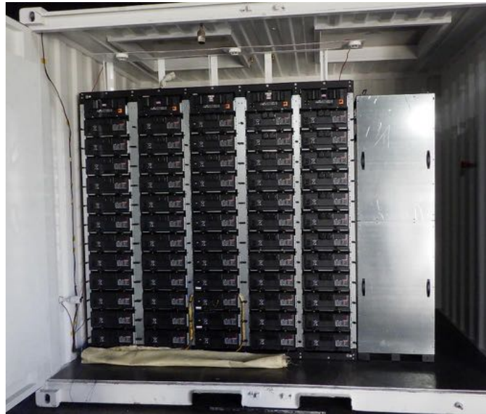
Figure 1 – Picture of the units in the container
