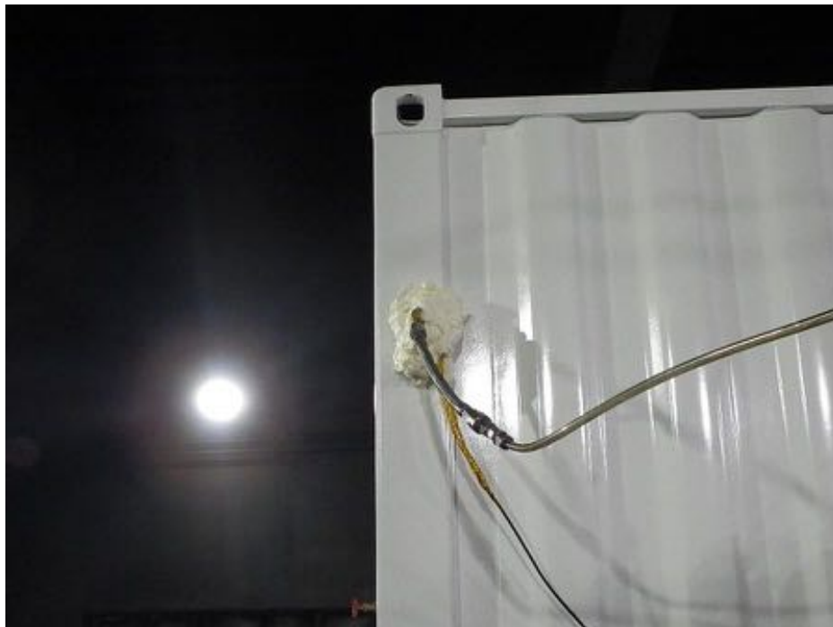
Figure F4 – Photo of the hoses going through the container wall and the urethane seal
