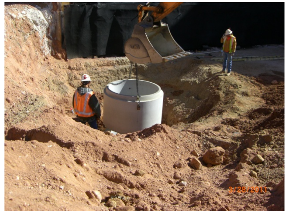
Sand/Oil interceptor north of lower basement
