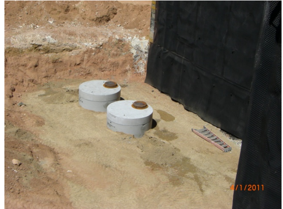
Sand/Oil interceptor north of lower basement
