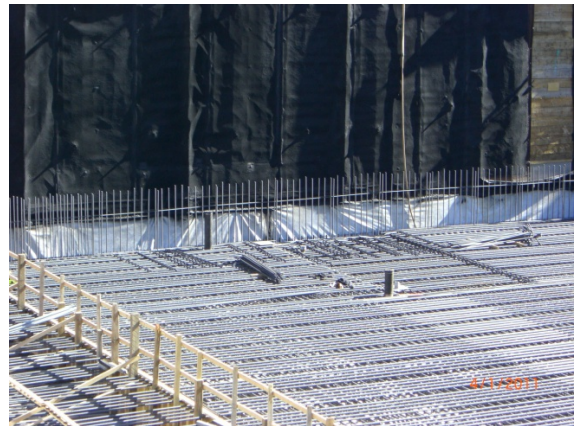
Close-up of rebar dowels for walls at east half of lower basement
